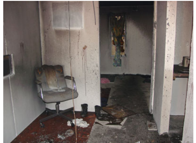
FIG. 8—View depicting locations saturated with water when the fire was extinguished, with “halo” effect evident against the back wall.
